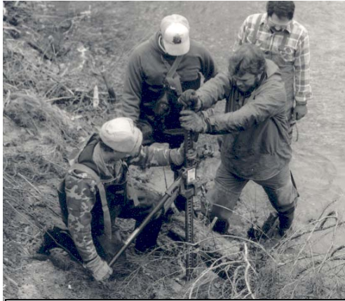
MDC stream biologists anchor a cedar tree, as part of a revetment at Young Conservation Area in
